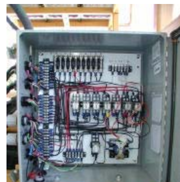
Figure 21: Electrical relay panel.
