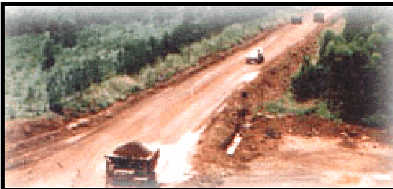
Connecting Road to Panchapattmali Mine Site. (No Plantation on both sides of road)
